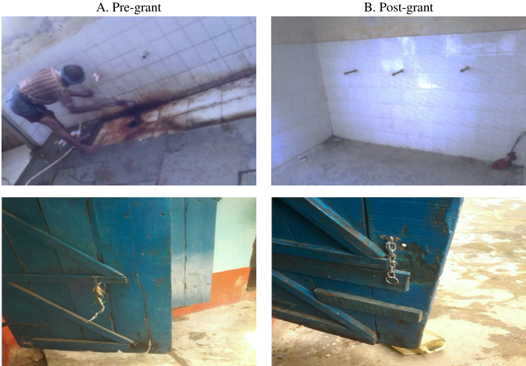
Note. Example of deep cleaning of walls and repair of locks in a CT in Lucknow. Panel A shows the status before the intervention, while Panel B shows the status after the deep cleaning. Source: Antonella Bancalari.
