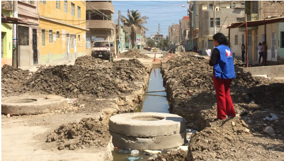
Figure A7 Abandoned Sewerage Project
