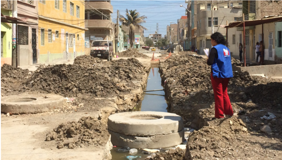
Figure A3 Sewerage project halted
